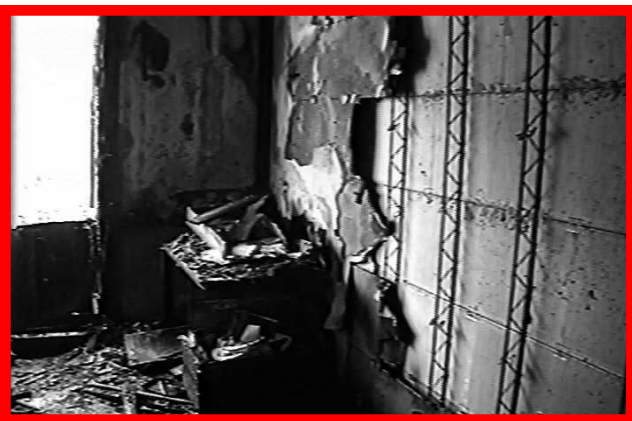
Resident room in Mathes after the 1997 fire.
