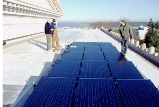
Photo 11: GA installed solar panels with the help of Puget Sound Energy. GA uses the panels to power the lights at the top of the dome of the
