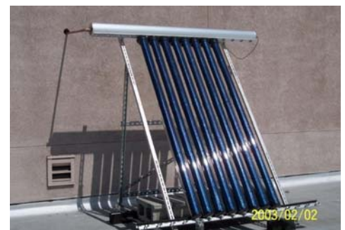
Photo 4: A Solar thermal water heating system installed by staff at Yakima Valley College.
