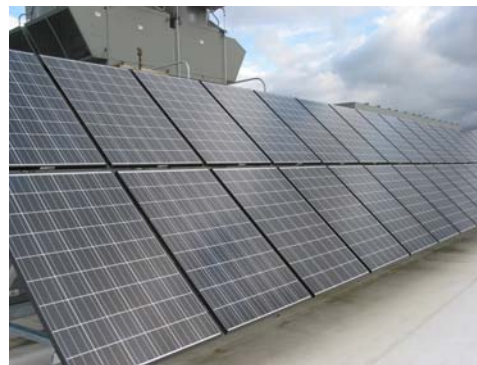
Photo 6: In the past year, Skagit Valley College has generated nearly 36,000 kwh from a Solar photovoltaic array on top of LEED Platinum Laura Angst Hall.
