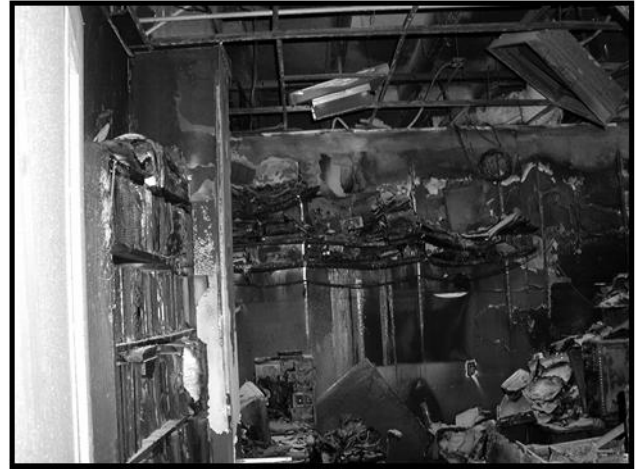
Parks Hall Fire— July 3, 2002 Destruction from an electrical fire related to computer equipment in Room 310
